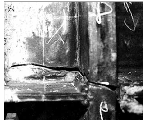
Figure 9: (a) Typical fracture initiation in Pre-Northridge beam-to-column connections in steel buildings; (b) Propagation of crack into the column flange and web. Photos courtesy of FEMA (FEMA-267: SAC Interim Guidelines and FEMA-350: Recommended Seismic Design Criteria for New Steel Moment-Frame Buildings, June 2000).
