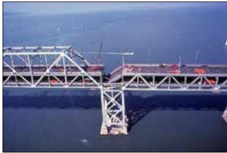
Figure 6. San Francisco Bay Bridge 2nd level collapse, Loma Prieta Earthquake (magnitude 6.9), October 17, 1989. Photo courtesy of USGS ( www.usgs.gov ).
