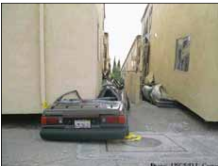
Figure 4. Soft story damage in a building during Northridge Earthquake (magnitude 6.7), January 17, 1994. Soft story is typically the result of one the stories being laterally softer than the others due to large window and door openings or parking garages. Photo courtesy of USGS ( www.usgs.gov ).
