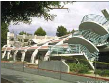
Figure 3. Severe damage in a concrete parking structure, California State University, Northridge, Northridge Earthquake (magnitude 6.7), January 17, 1994. Photo courtesy of USGS ( www.usgs.gov ).
