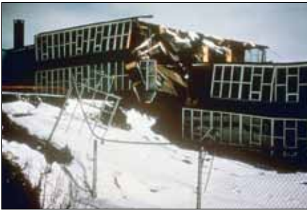
Figure 2. Damage due to ground deformation in a school in Anchorage, Alaska Earthquake (magnitude 9.2), March 28, 1964. Photo courtesy of NGDC ( www.ngdc.noaa.gov ).
