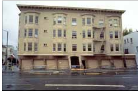
Figure 5. Soft story damage in a building during Loma Prieta Earthquake (magnitude 6.9), October 17, 1989. Photo courtesy of USGS ( www.usgs.gov ).
